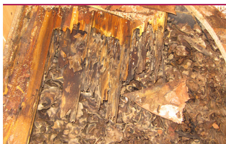
Orange ants - decomposed floorboards. (Photo: Protox/customer photo)
