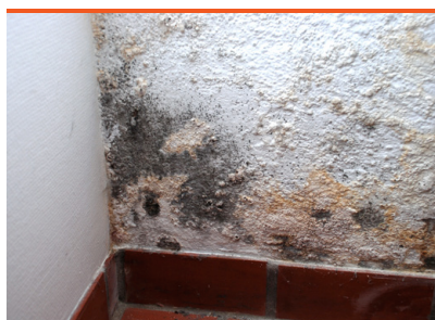
Mould infestation in basement
