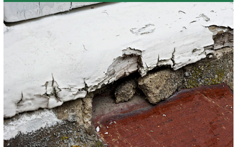
Surface rot (grey rot) – dripping on old window. (Photo: Prottox)
