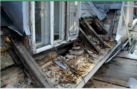
General advice – eaves broken down. (Photo: Tryg Forsikring)
