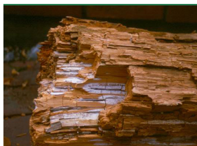
Mine fungus – crack bricks. (Photo: Goritas)
