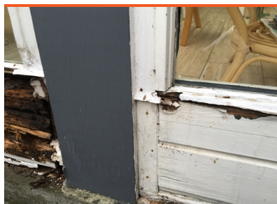
Window section with clear fungal attack
