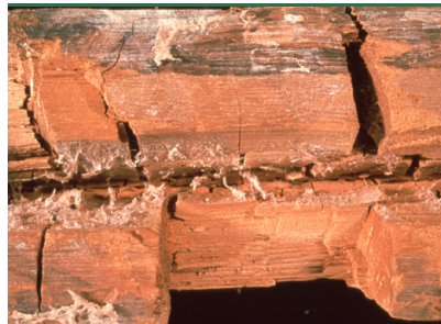
Dry rot fungus- crevice blocks. (Photo: Protax/Gori)
